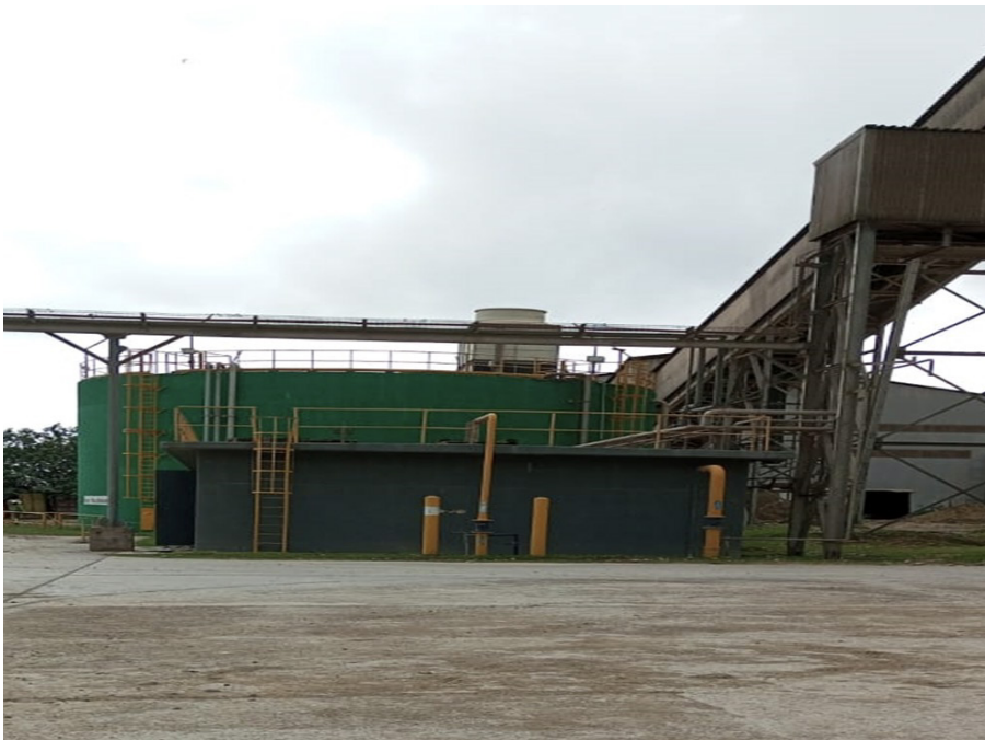
Ewekoro water recycling installations.
