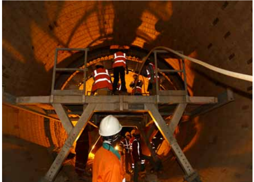
An engineering team working in the kiln in WAPCO Operations' Ewekoro Line II plant.
